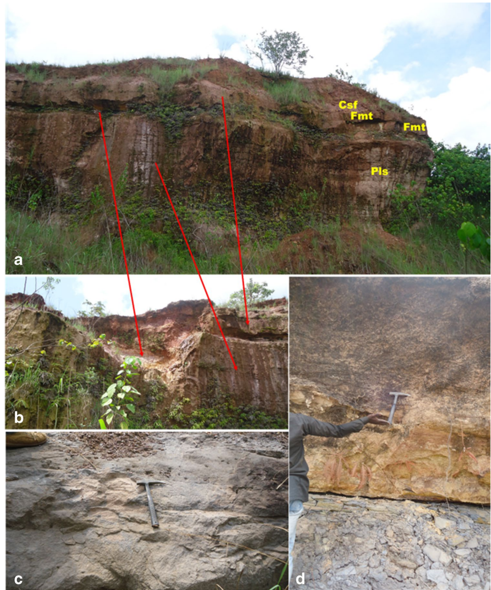
Fig. 3 a An overview of the outcropping section at Ikpankwu depicting a general oscillating depositional sequences of fining and coarsening upward sequences. b Normal fault system showing fault-bedded horizon of the Ikpankwu outcrop displaying reddish brown to pink claystone facies (Csf), plane planar laminated sandstone facies (Pls) and consolidated siltstone facies (Fmt). c Consolidated structureless sandstone facies (Smc1). d Carbonaceous black shale facies (Shfc) of the Nsukka Formation overlain with sharp contact by a partly consolidated fine-grained sandstone to siltstone facies
