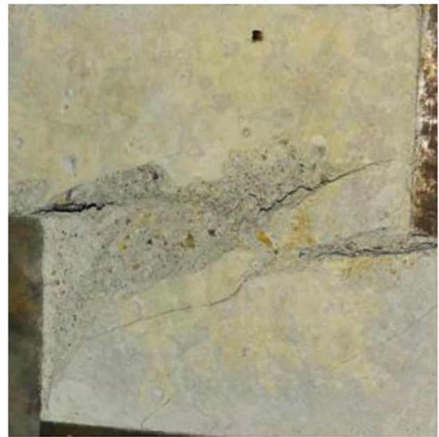
Fig. 11 Fracture morphology of the specimen with a crack length of 0 mm
