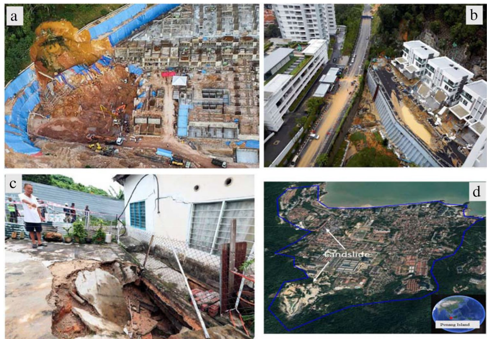
Fig. 1 Field photographs showing various ground deformations: (a) depicts a landslide scar on 67° slopes at Tanjung Bungah, (b) represents a collapsed retaining wall protecting the road at a newly completed housing area built on a hillslope, at Tanjung Bungah, (c) shows subsidence event in Mount Erskine, near Tanjung Bungah (Chacko 2019), and (d) denotes photograph of the slide area overlaid to a Google Earth image
