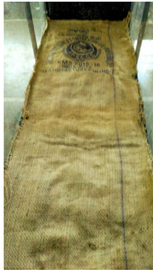
Fig. 6 Placing of jute geotextile as a separator between drainage layer and soil
