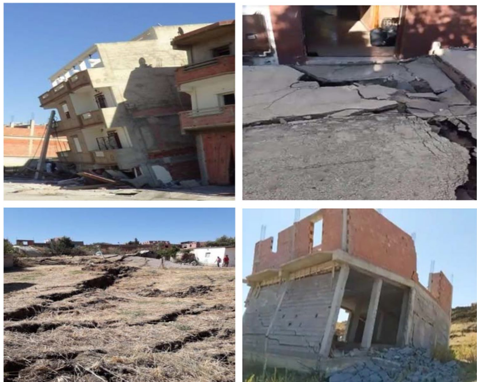
Fig. 6 Damage observed by landslide caused by earthquake in Mila region
