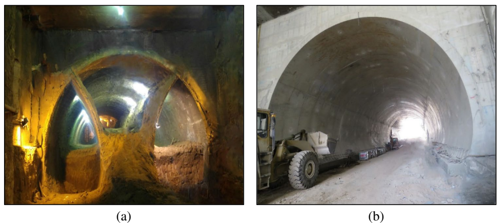
Fig. 7 Main support systems in studied case: (a) composite support system (b) final lining
