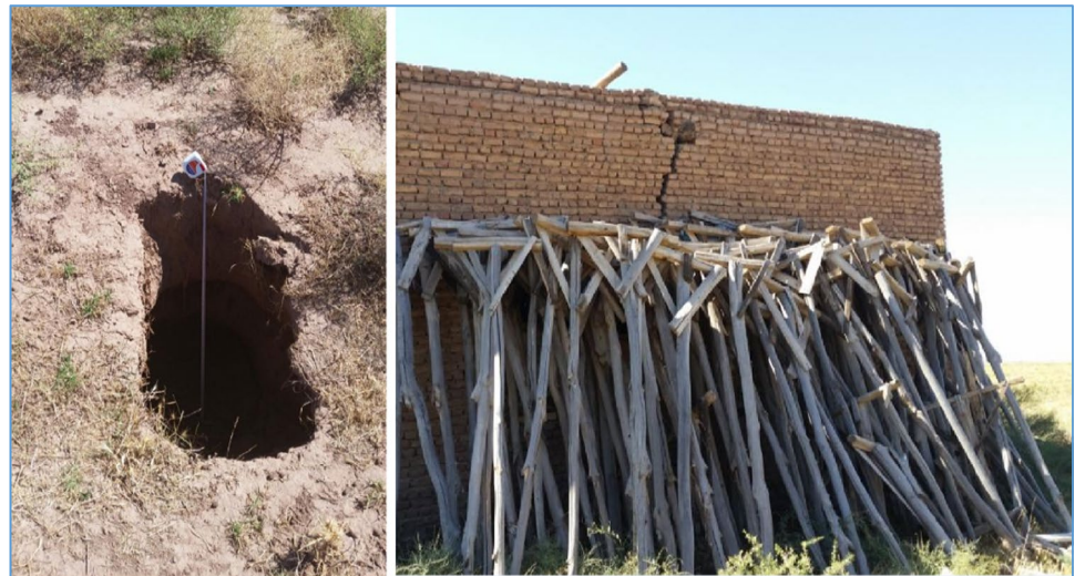
Fig. 5 Sinkholes and damaged buildings due to land subsidence (September 2015)
