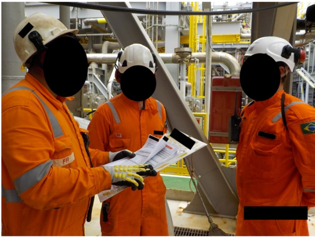
Fig. 10 Interaction with a maintenance team in the oil treatment external area. Source: Authors (2020)
