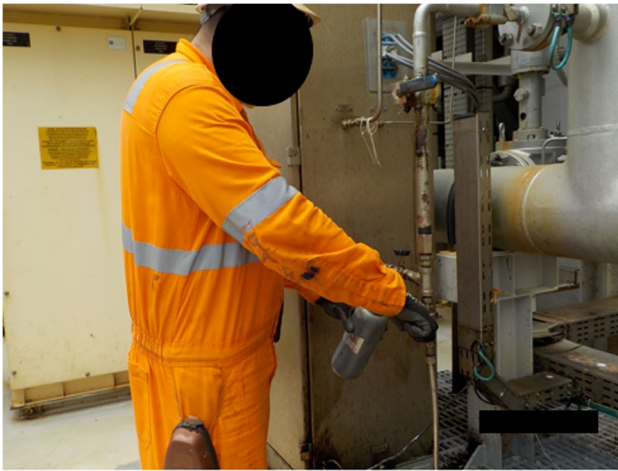
Fig. 2 Operator performing an oil sampling operation in the process plant. Source: Authors (2020)
