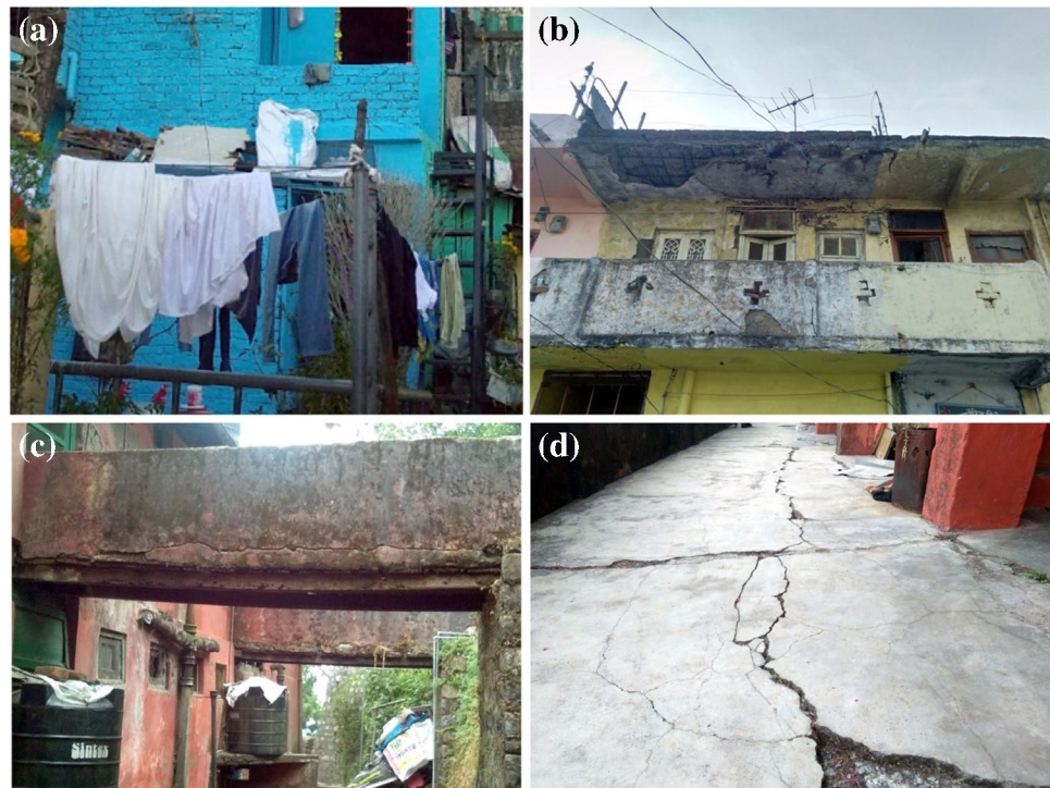
Fig. 8 a Field photograph of building ID: H24 ( R : 0.48, SSV class: III); b field photograph of building ID: H37 ( R : 0.63, SSV class: II); c, d field photograph of building ID: H43 ( R : 0.64, SSV class: II)
