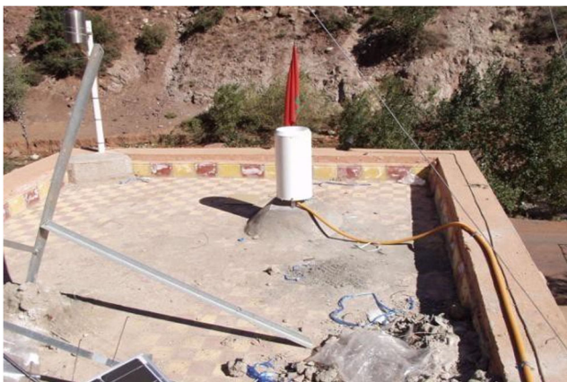
Fig. 6 Tipping bucket rain gauge
