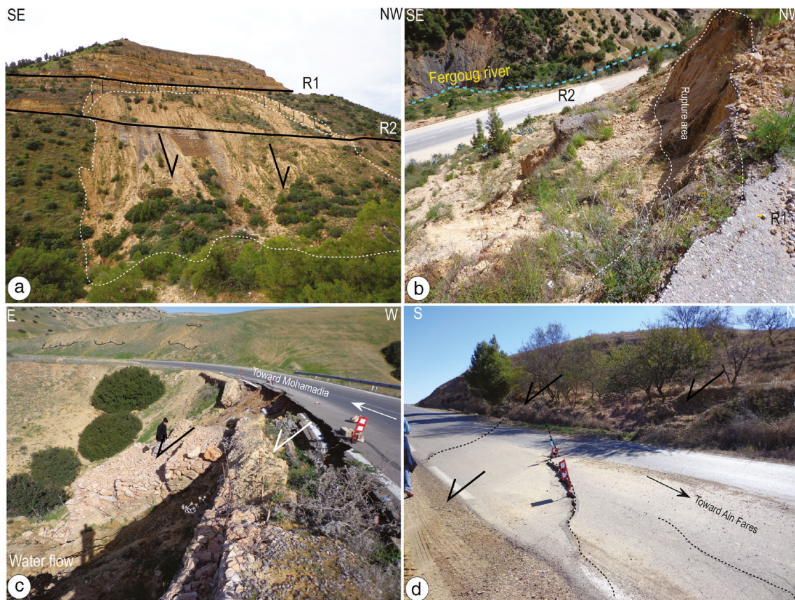
Fig. 3 Roads affected by landslides in different location, a: road connecting Mascara to Mohamadia affected as a whole by a large landslide (dark line represents the road which leads from Mascara to Mohamadia), b: the landslide seen from one top, the dashed lines show the limits of the landslide area, c: the cliff corresponds to the rupture zone, even the device designed to protect the road was affected by the great
