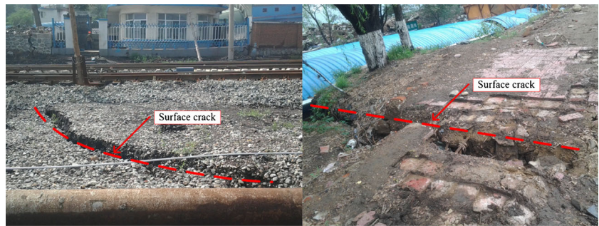
(a) the surface crack
