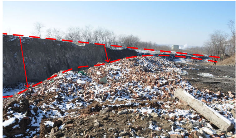
(b) the tensile crack in the top of the slope
