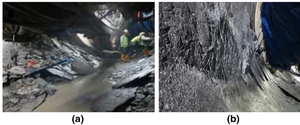
Fig. 6 Rock overstepping at the Pahang Selangor Raw Water Tunnel a at 1050 m (Ch. 16,300 m), b at 130 m (Ch. 24,610) (Azit et al. 2015)
