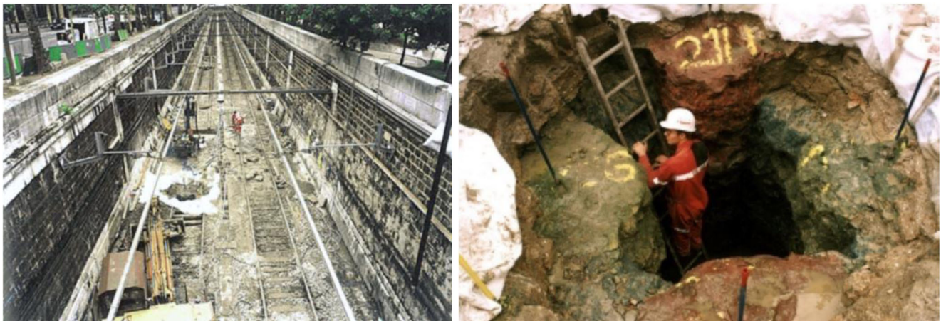
Fig. 16 View of the on-site trial and the grouted columns obtained from the trial test (source: http://www.soletanche-bachy.com )
