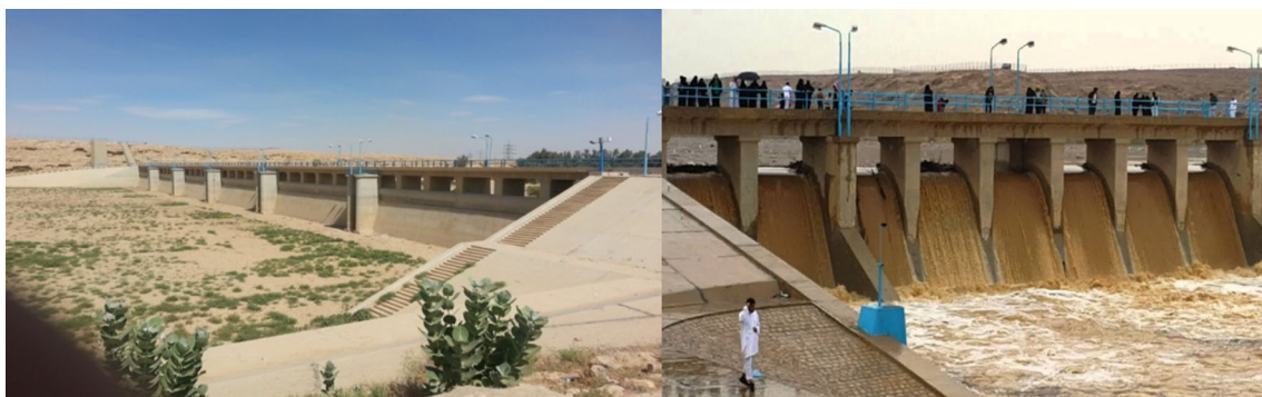
Fig. 8 Images of Al-Ulb dam in Riyadh Region, left image: upstream of the dam during the dry season showing empty reservoir and upstream face of the spillway; right image: flow over the spillway during a recent flood on November 25, 2015 and downstream channel flow
