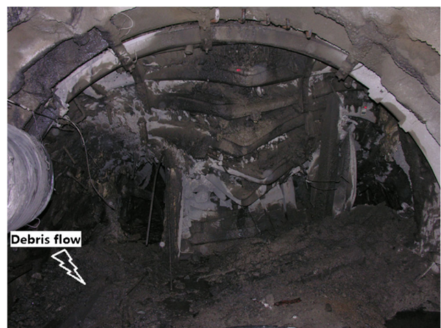
Fig. 7 The roof collapse and debris flow at the tunneling face near fault FD108
