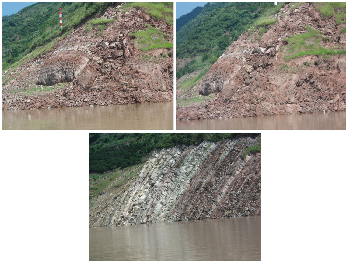
Fig. 12 Typical failures of red-layer soft rock in the vicinity of hydro-fluctuation belt in Three Gorges reservoir area (July 2013)
