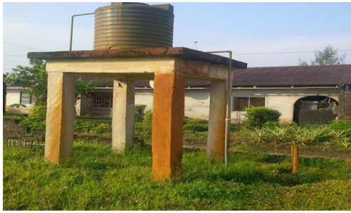
Fig. 20 A picture showing a typical abandoned borehole with corroded rubber tank, raised concrete platform, and plastic pipes due to contamination of aquifer near VES 5
