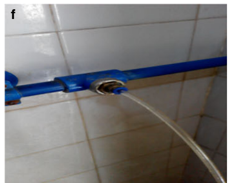
Faucet connected to device (c)
