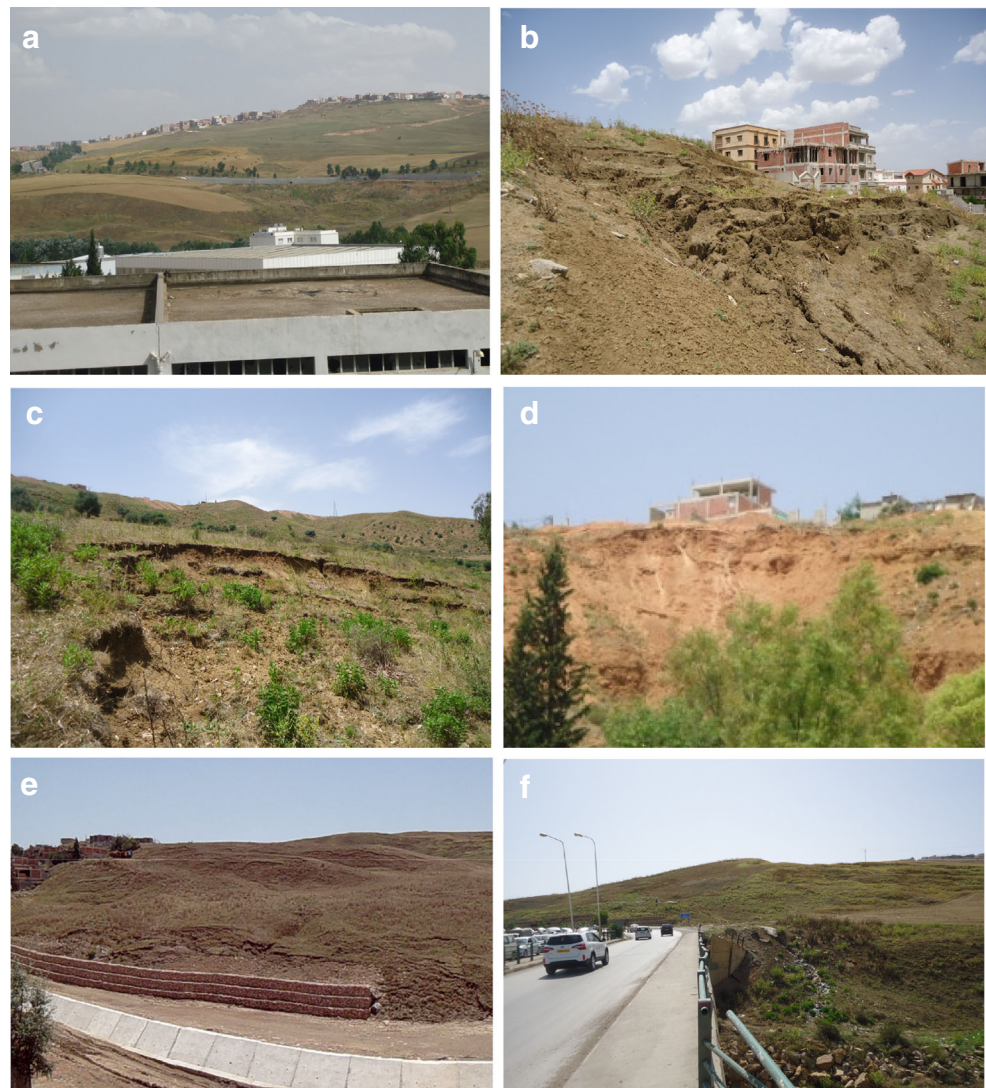
Fig. 2 Field photographs showing the characteristics and types of recently occurred landslides in the study area: a rotational slides over the road of Massinissa, b rotational slides in Boussouf, c rotational slides along road in Benchergui, d fall slides in Benchergui, e rotational slides in Chabet El Merdja, and f rotational slides of the Rhumel bridge in Massinissa
