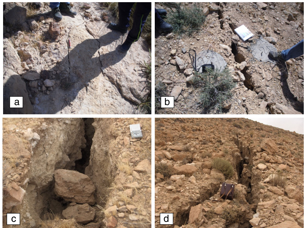
Fig. 3 a, b, c Photos showing the width of the cracks. d Overall view of the crack extending more than 280 m
