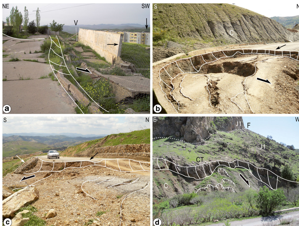
Fig. 4 Photographs showing different types of landslides. a Landslide (L5) affecting a stadium and another building below, V vertical line reference, black arrow showing a wall destroyed and partly tilted; b road affected by landslide (L41) west of the Grand Pic isolating people living in the other side; c landslide (L12) southwest of Belkheiret affecting colluviums deposits and damaged a new road build 3 years
