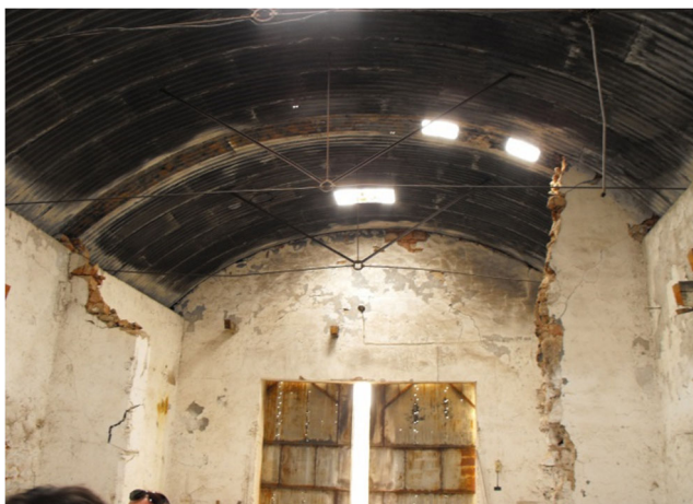
Fig. 18 Current view of the original roof in a warehouse at La Tortilla smelting works
