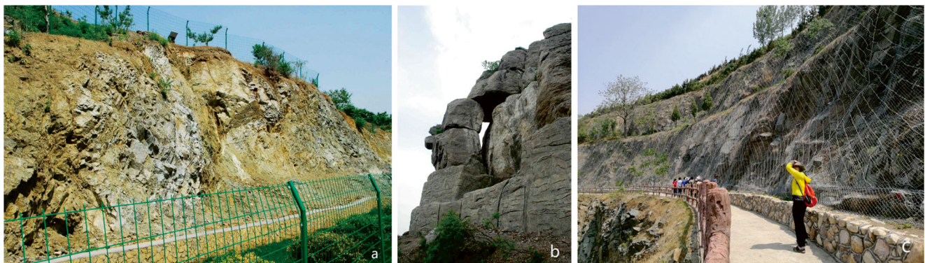
Fig. 9 Geohazard protection. a Geohazard surrounded by a fence. b Fissures reinforced by anchor and injection. c Slope reinforcement
