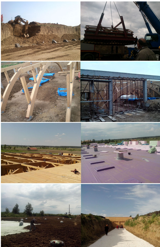
Fig. 6 Construction process of the protective structure in The Mammoth Park. Photos: Institute of Archaeology Belgrade
