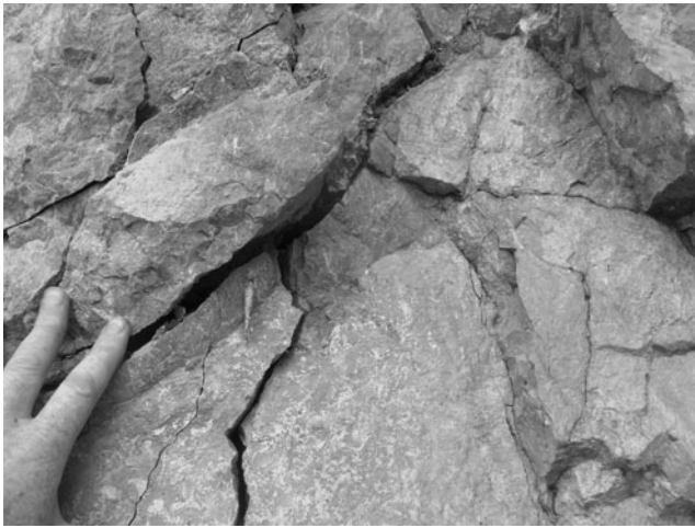
Fig. 18 Destabilised rock faces that surround the mouths of shelled caves such as Tham Piu highlight the fact that not all the damage caused by war has yet run its full course, and that further cave collapse and the implications of changed natural process pathways inevitably persist long after active combat has ceased
