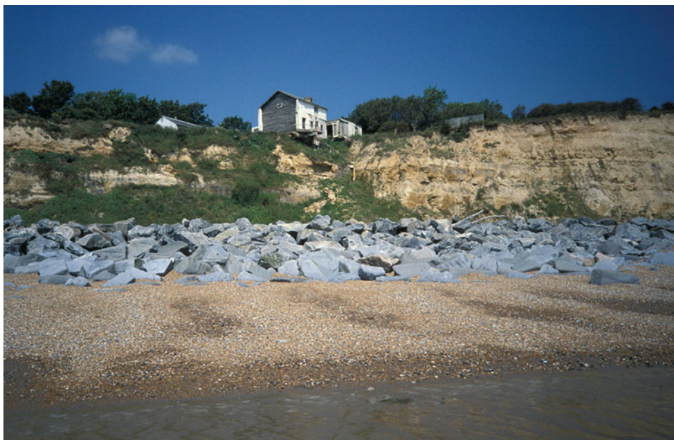
Fig. 4 Eroding cliff exposures, Fairlight Cove, East Sussex, England, threatened by the human response to climate change. Blocks of rock used as ‘hard’ coastal protection are starting to result in slowed erosion and degradation of the exposures. Photograph: Jonathan Larwood/Natural England
