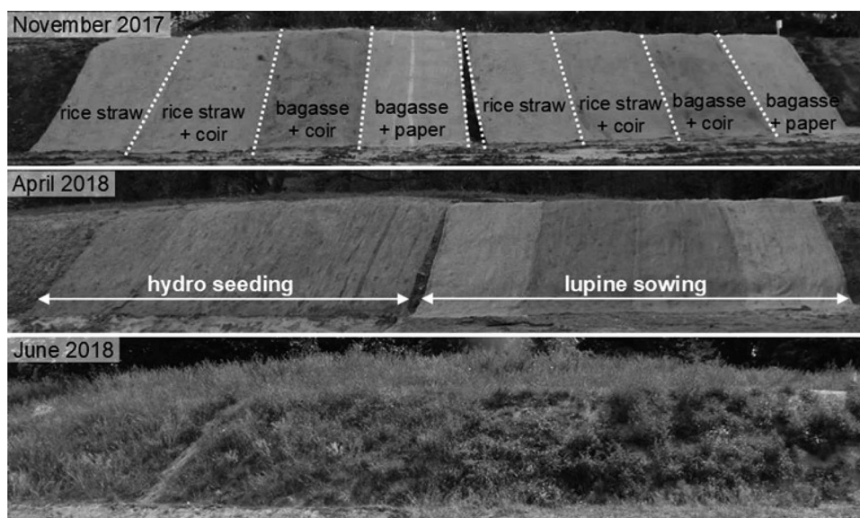
Fig. 4 ECBs from Vietnam sugarcane bagasse and agricultural by-products during the trial at construction site at TU Bergakademie Freiberg (2017–2018) (Katja et al. 2020)
