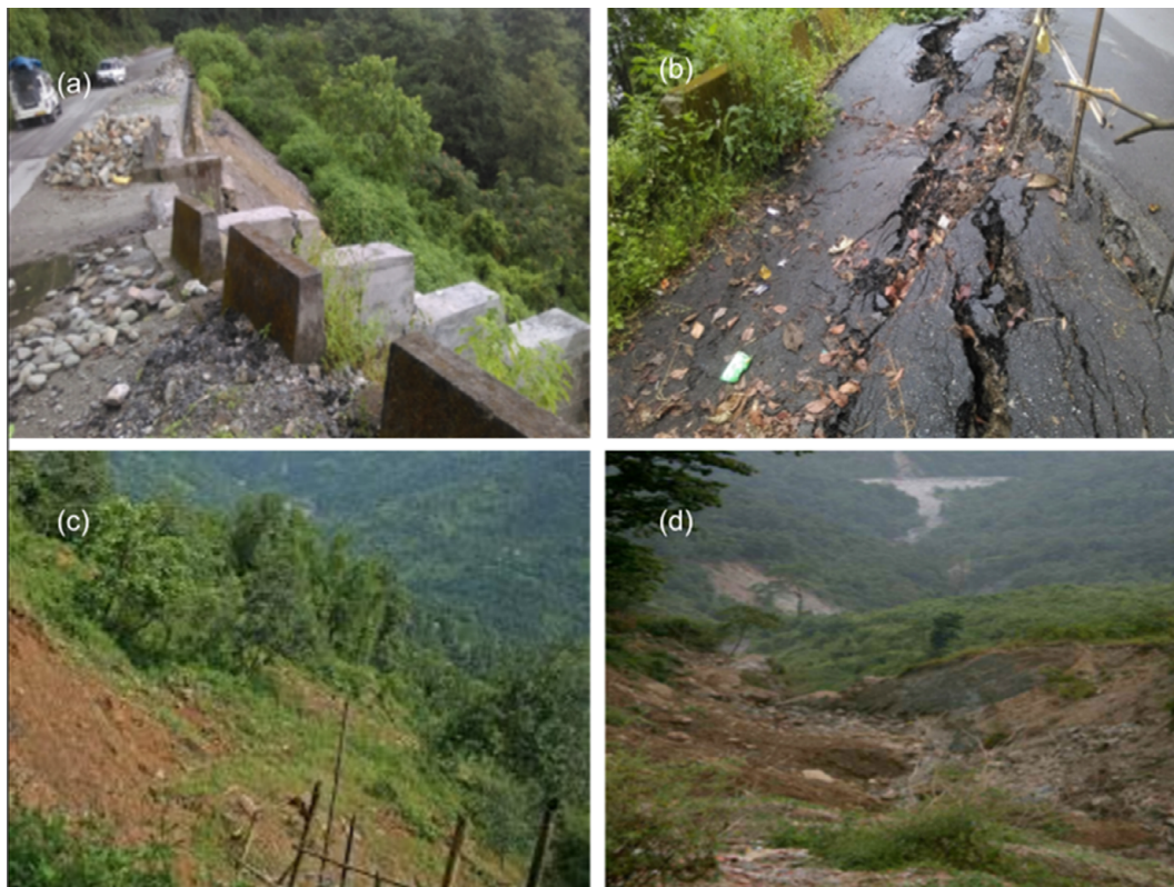
Fig. 3. Landslide damages in the region. (a) Damage to culvert, (b) Damaged road section along NH-31A, (c) Land loss during 2015 landslide event, (d) Mudflows and debris (2011 event) ( https://savethehills.blogspot.com ).
