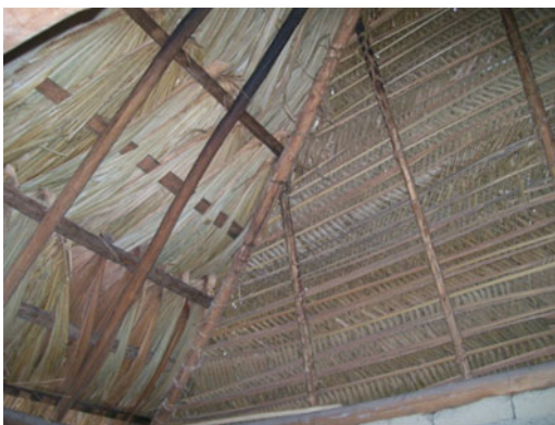
Fig. 2. Roofing of a Kalunga home; the right side is covered with indaiá leaves, the left side with buriti leaves. Engenho II, Cavalcante-GO.
