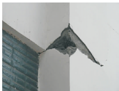
(b) Damage of a column end
