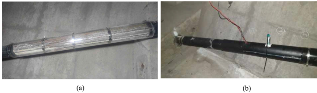
Fig. 1. Field Experiments on Corrosion Tendon Repair (KIBSE, 2020): (a) Long-term Observation without Grout, (b) Long-term Observation with Grout Reinjection
