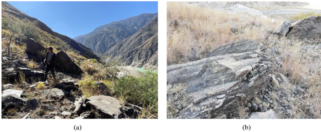
Fig. 3. Buckling on Landslide: (a) Curved Uplift Phenomenon of C Area, (b) Uplift and Fracture of Rock Layer in D Area
