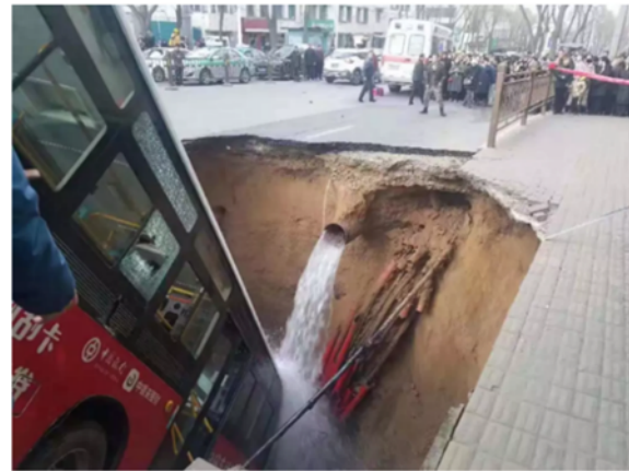
Fig. 2. Road Collapse Accident in Xining City
