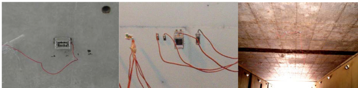
Fig. 6. Sensors on Taxiway Bridge V
