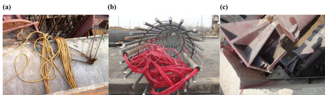
Fig. 4. Pictures of In-situ Monitoring: (a) Wall Deflection, (b) Rebar Force, (c) Bracing Force
