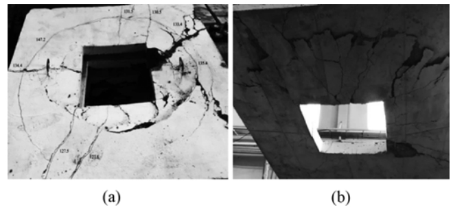
Fig. 8. The Failure Mode and Cracking Pattern for Slab SOM: (a) Compression Side, (b) Tension Side
