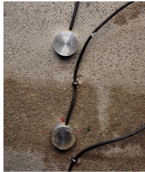
Fig. 3. Water Pressure Sensor
