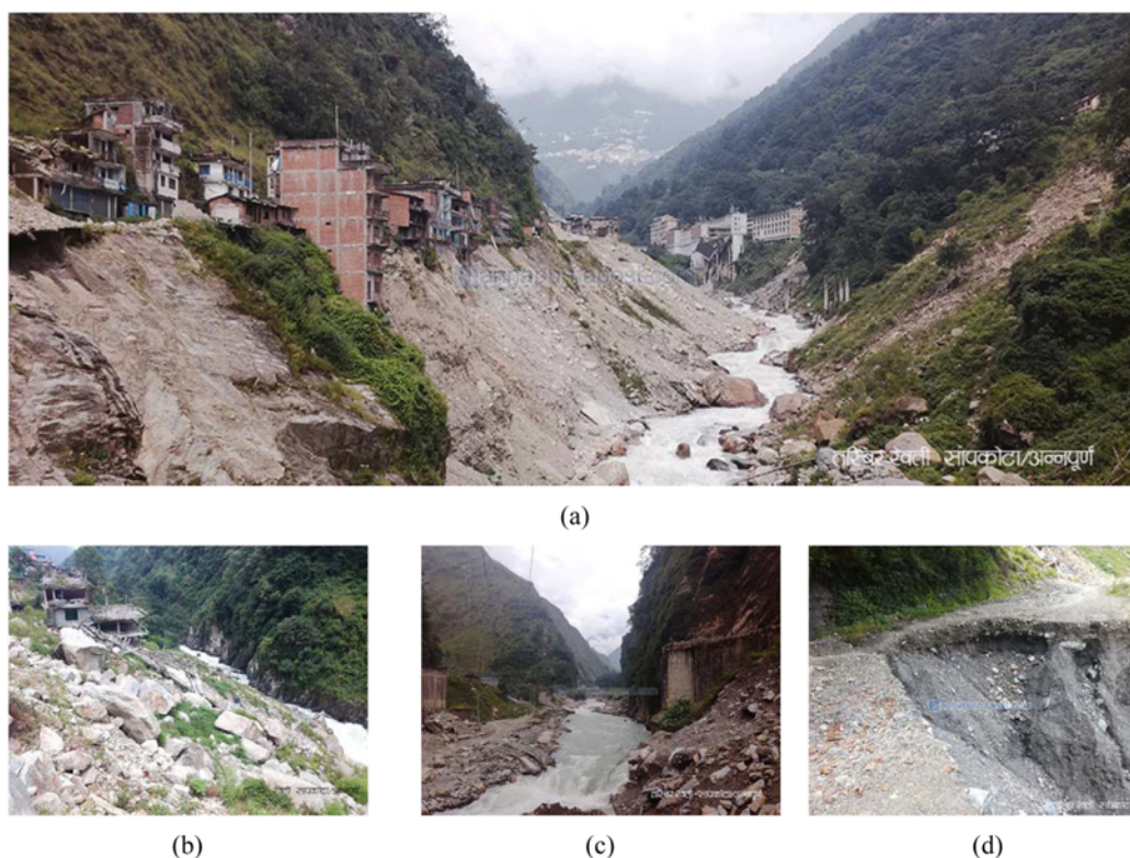
Fig. 8. Situation of the Araniko Highway after Earthquake (Sapkota, 2017): (a) Tatopani Bazar, (b) Bhote Koshi River Bank, (c) Phulping Bridge, (d) Damaged Road
