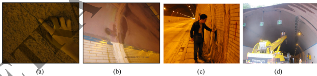
Fig. 3. Damages Investigation and Detection for Hui-long-shan Tunnel: (a) Lining Cracks, (b) Lining Seepage, (c) Lining Breakage, (d) GPR Scanning
