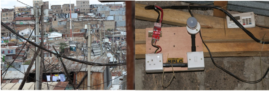
Fig. 4 Electrical connections in the settlement (source: authors)
