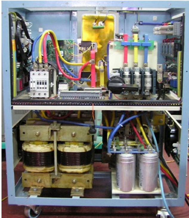
Figure 6. Shunt HAPF assembled in a panel.
