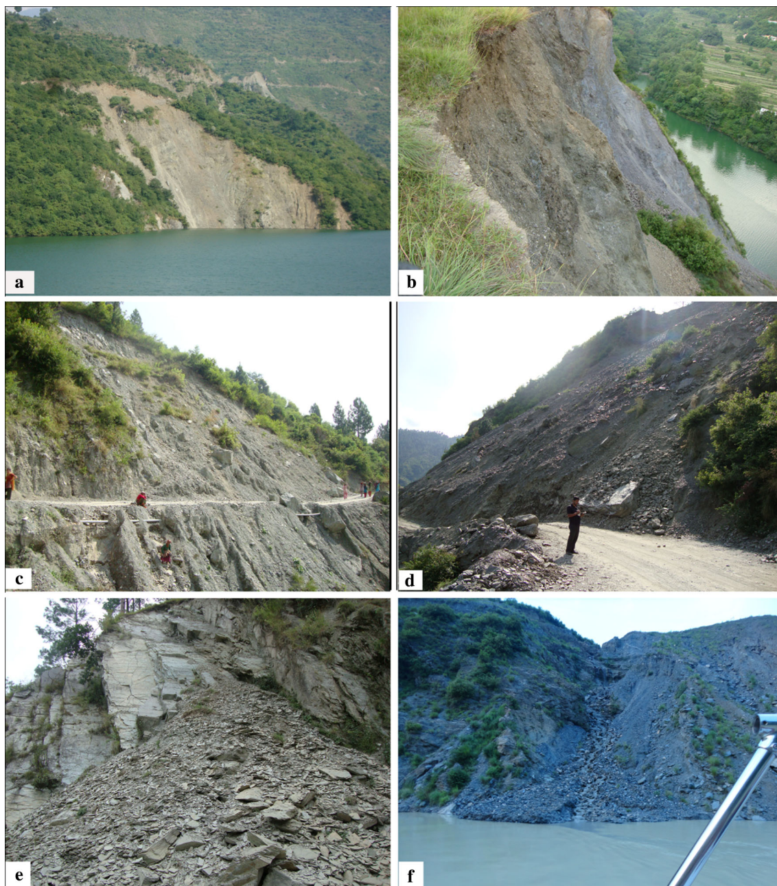
Figure 3. Field photographs: (a) typical arcuate shape scar of the reservoir-induced landslide, (b) slope failure in RBM, (c) rotational failure along the road network, (d) rotational failure in debris along the road and (e) slope form of phyllite is subjected to plain failure and (f) drainage-induced landslide.
