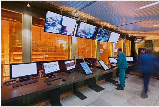
Fig. 5 Operator control pulpit (courtesy of Danieli Automation)
