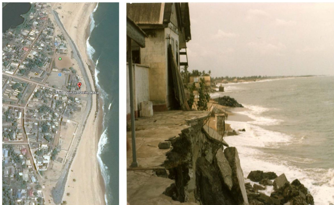
Fig. 5 Left: Visible beach area, building with sea defense system at Fort Prinsensten, Keta. Right: Massive erosion with no beach and property loss at Prinsensten, Keta in 1985, Ghana
