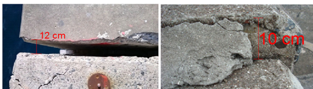
Fig. 2 Damages visually identified
