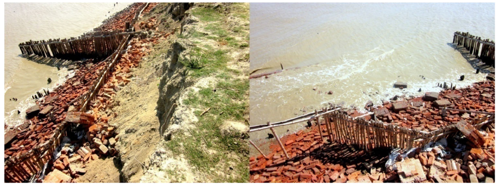
Fig. 7 River bank erosion in Muriganga estuary (eastern part of the Sagar Island)
