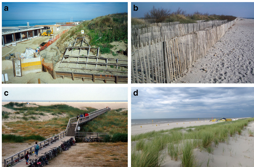
Fig. 6 a Trench in the dune system to give access to new bath houses on the Tuscany coast (Italy); b Sand fences at Montpellier (France); c Dune walkway in Denmark; d Dune vegetation planting (The Netherlands)
