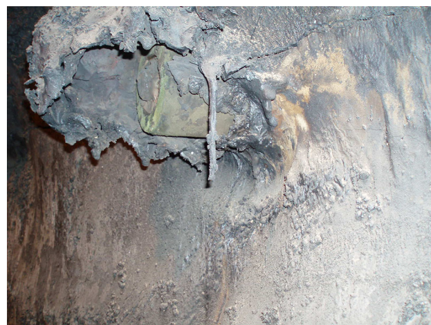
Fig. 5. Oxygen lance. Massive build up and wash outs of the refractory side wall below the build up.
