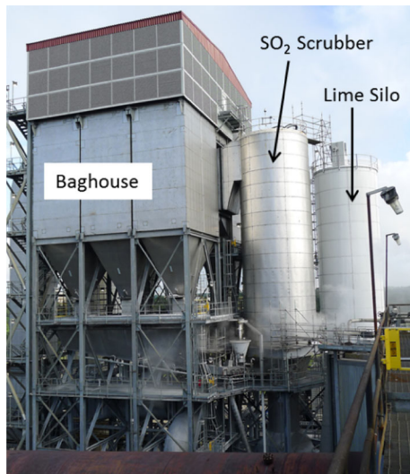
Fig. 17. Baghouse, SO 2 scrubber, and lime silo (L to R) at Lake Charles calciner.
